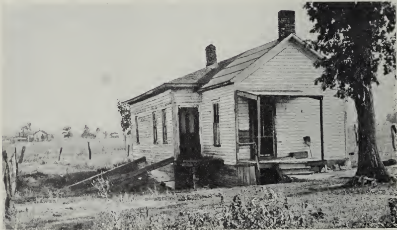
FIG. 45.—Small house near Streator beside which a pit hole 10 by 20 feet and 5 feet deep has formed.
